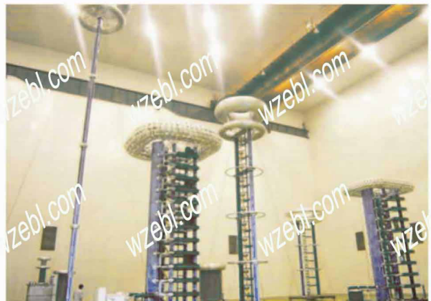
H.V Testing Hall
